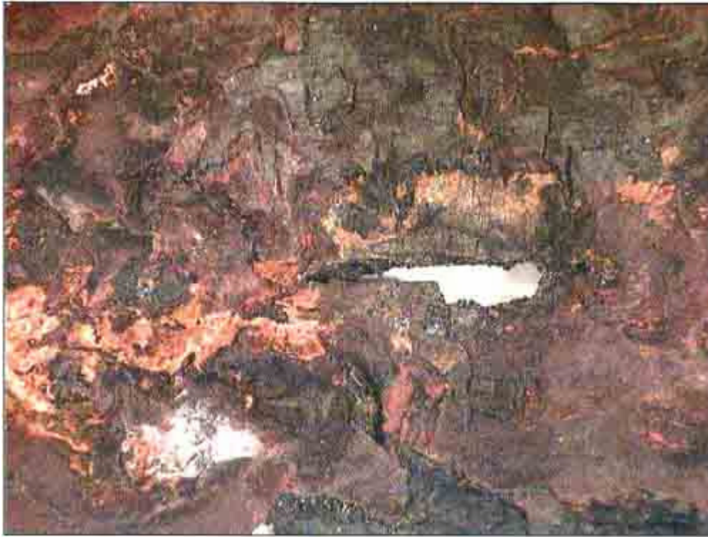
FIGURE 43 - Photograph showing the perforation in the tube wall thickness at the ID surface.
