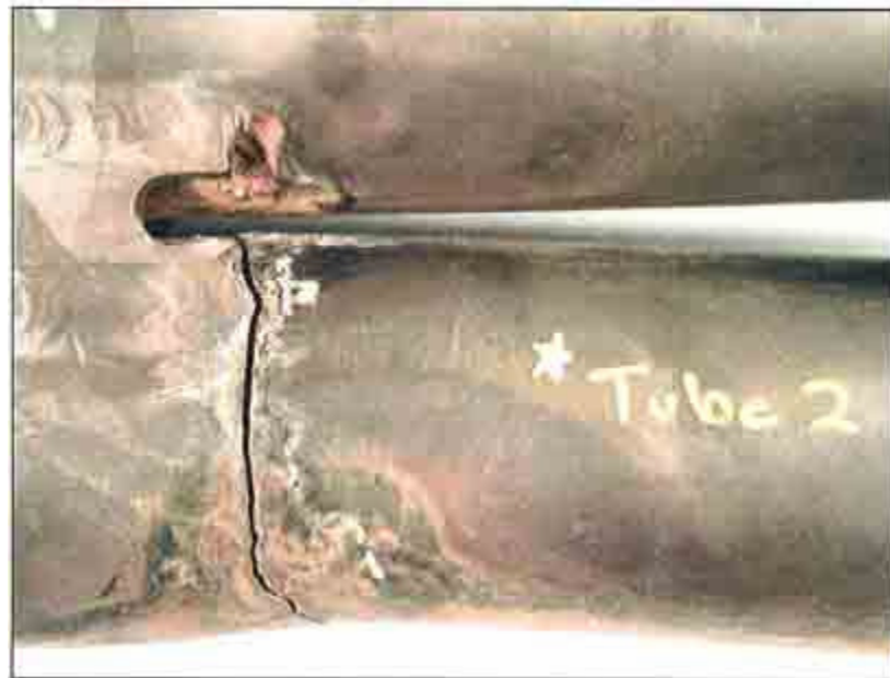
FIGURE 2 - Photograph showing the circumferential crack in tube no. 2.
